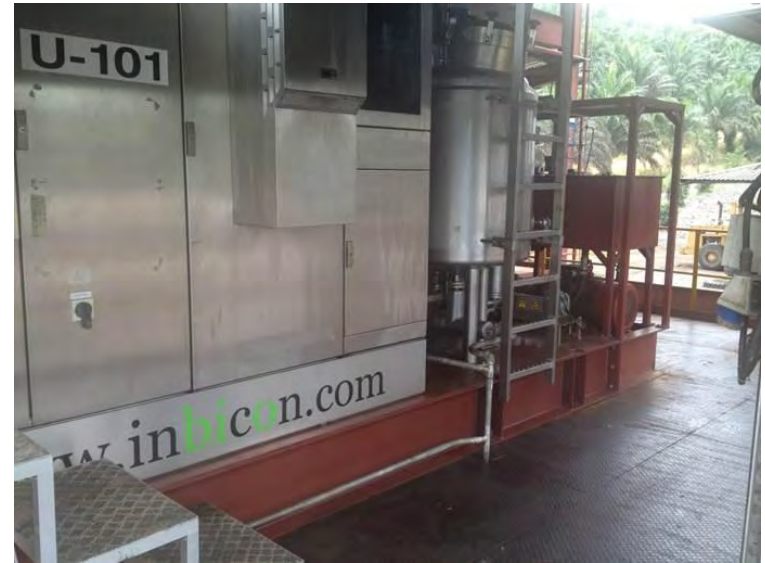
Pilot plant operating in Tawau, East Malaysia. Converts empty fruit bunches into 2nd generation bioethanol. The project is part of an on-going collaboration between Inbicon, Mitsui Engineering & Shipbuilding and Teck Guan.
